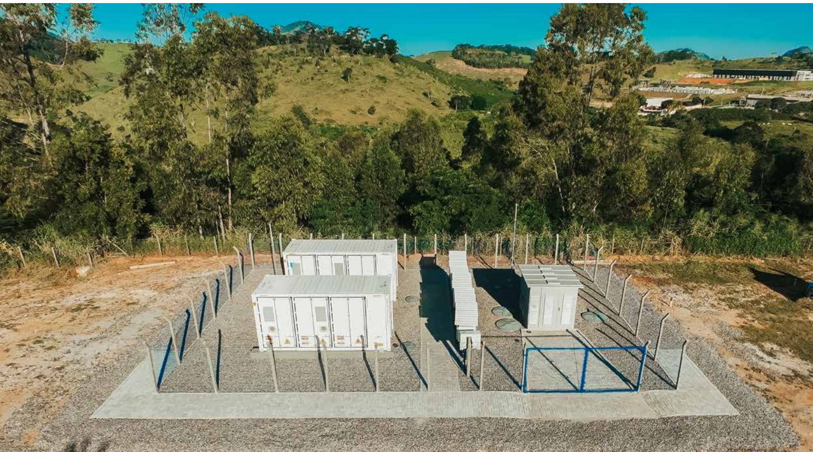
Matrix Energia's projects incorporate Huawei's battery energy storage systems.
