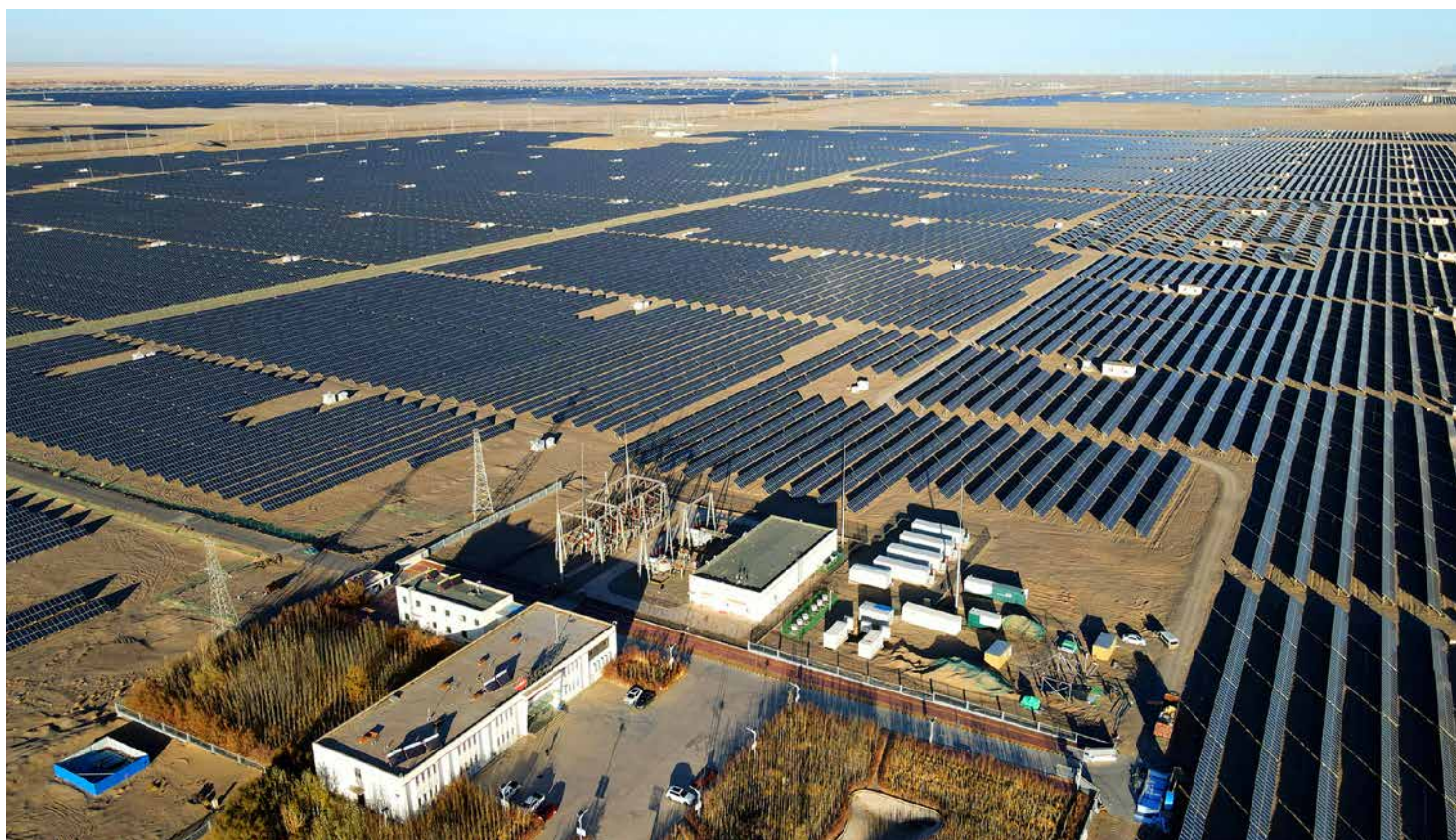
The Golmud project supplies 1 MW/2 MWh of energy storage for the grid in Qinghai, China.
