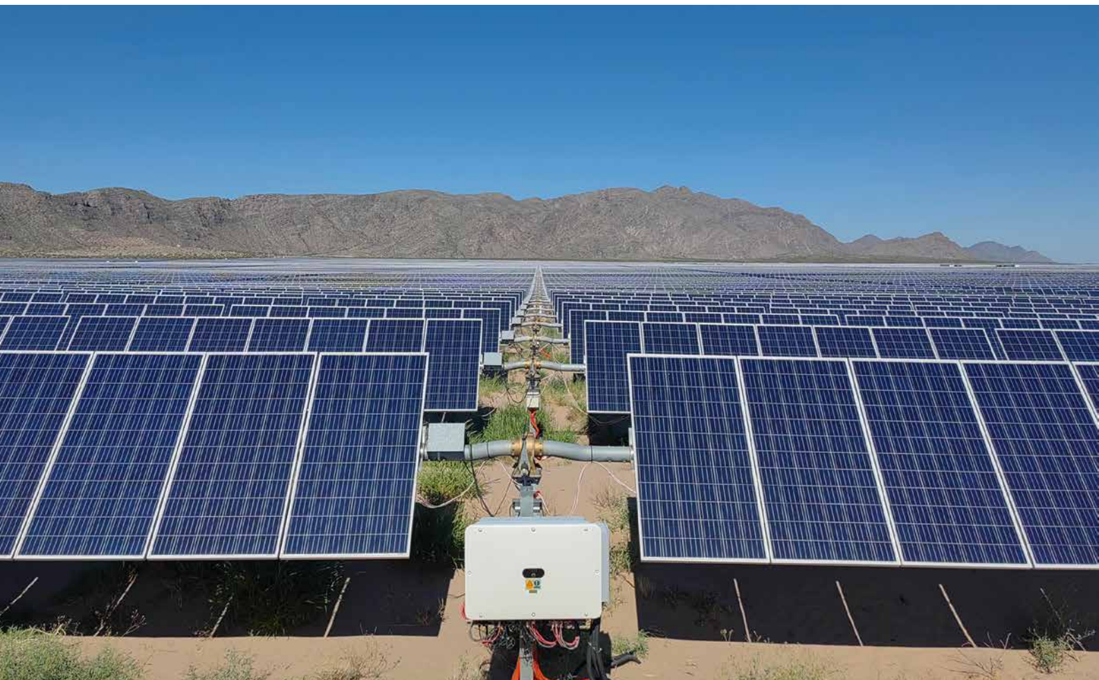
Huawei's string inverter technology is used at Kino Energia's Villanueva project.
