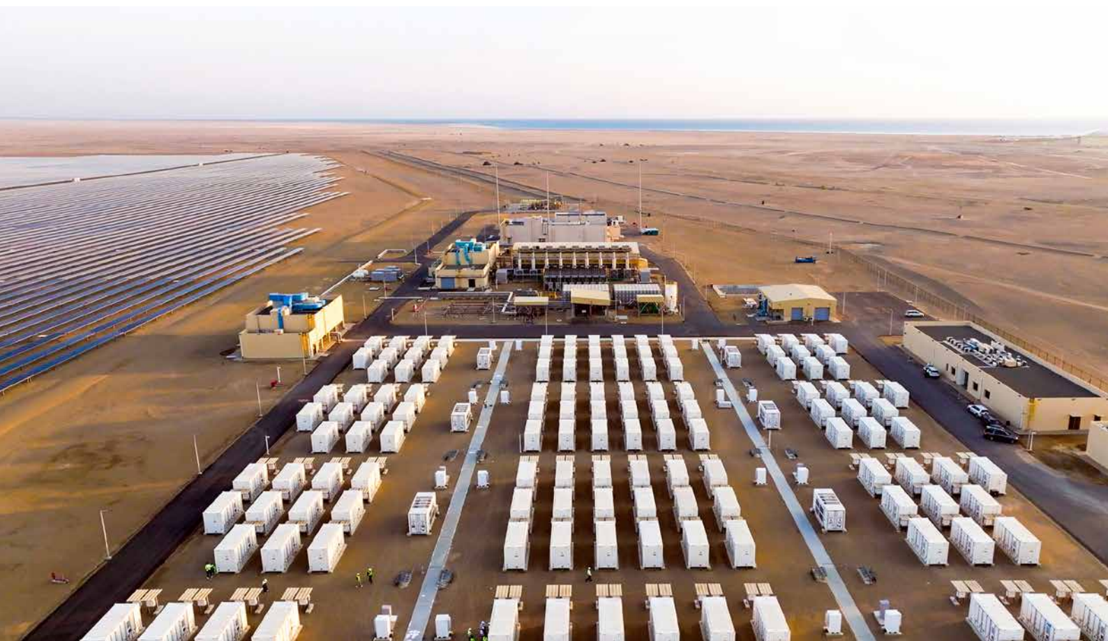
Huawei's Smart String Grid-Forming ESS Solution supports the solar PV microgrid for The Red Sea destination.
