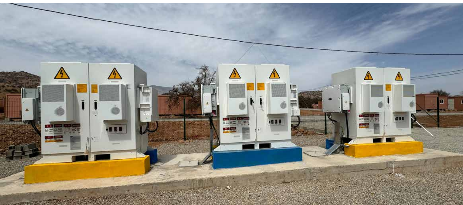
MASEN uses Huawei's LUNA2000 energy storage solution in its microgrid projects.
