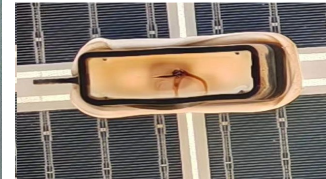
Burnt and damaged junction box
