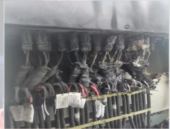
Frequent terminal burning faults
