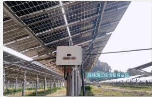
Reverse connection of PV strings
