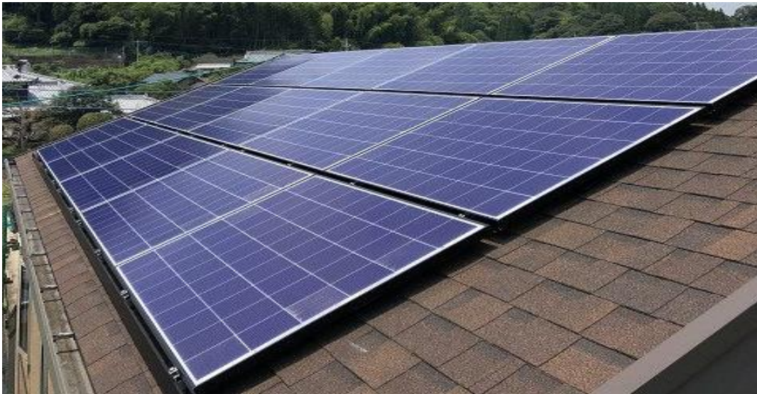
Residential modules in Osaka, Japan (installed in 2014)
